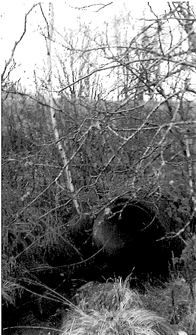
Figure 4-1: Stream from south passing the road in culvert (Reference). Road can be seen above.
