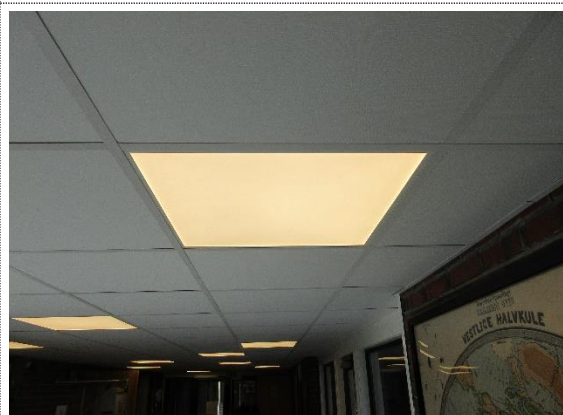
440.01 Nyere type LED armaturer for systemhimling
