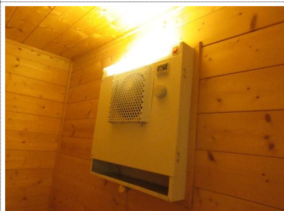
610.01 Aggregat for kjølerom
