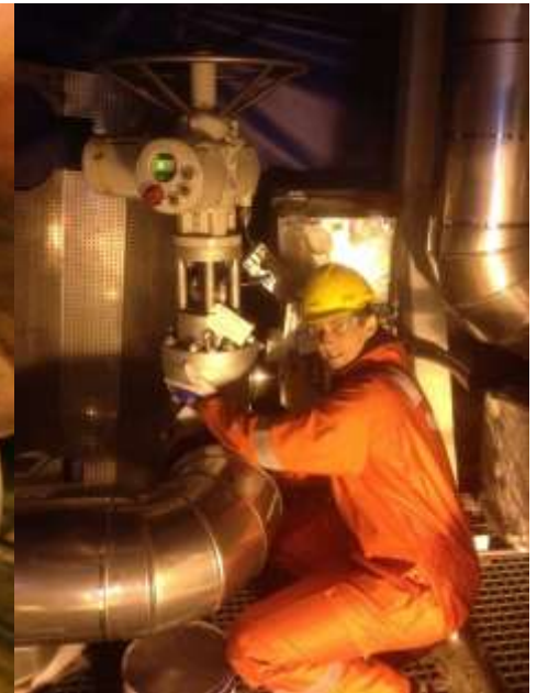
On site inspection – Kværner Stord, EG 6"300lb Double Expanding Gate c/w Electric Actuator
